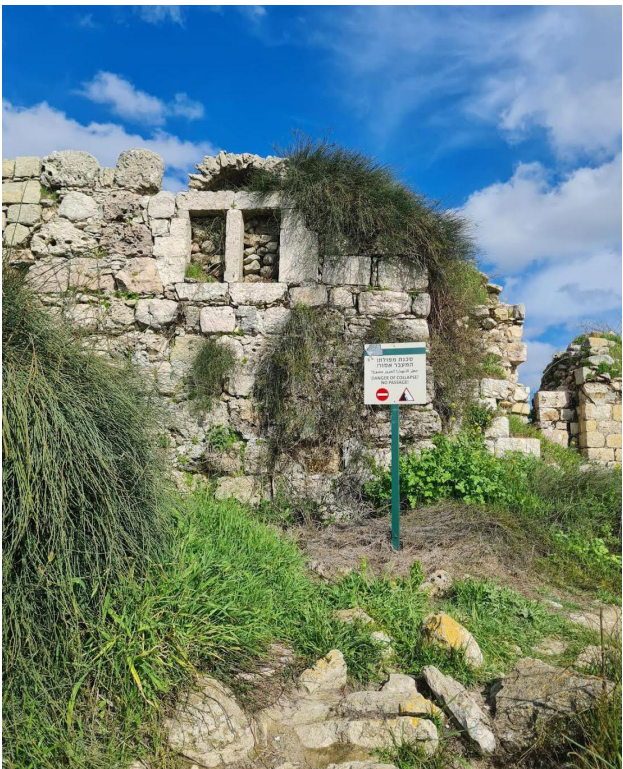
Palestine landscape with sign saying “Danger of collapse, no passage!” Courtesy of Rawan Nemer.
